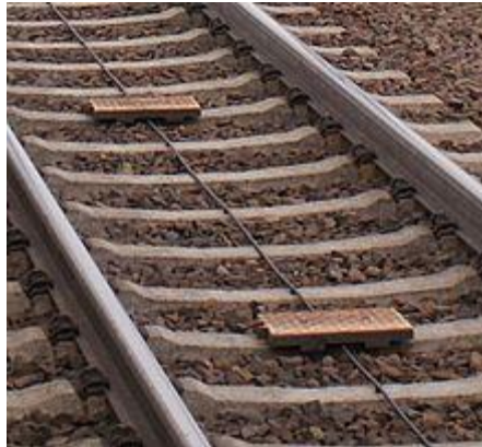
Figure 2: Balises along the railway track
